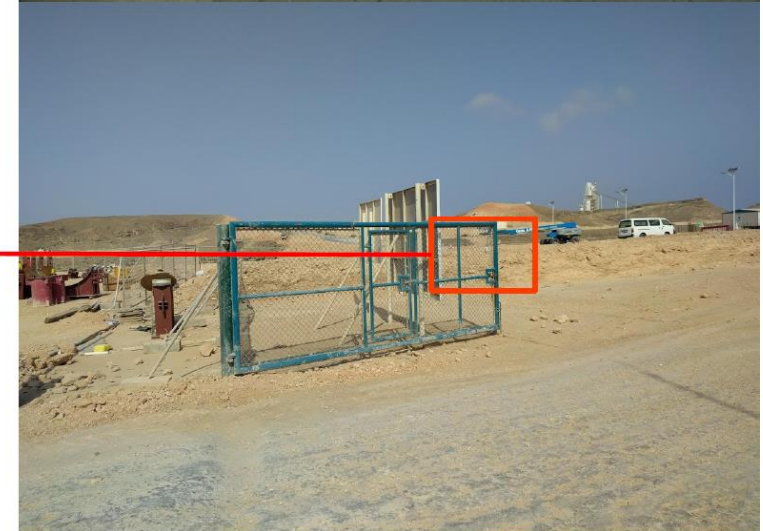
Bluetooth beacons hooked to an entrance gate to detect site entry / exit by car
