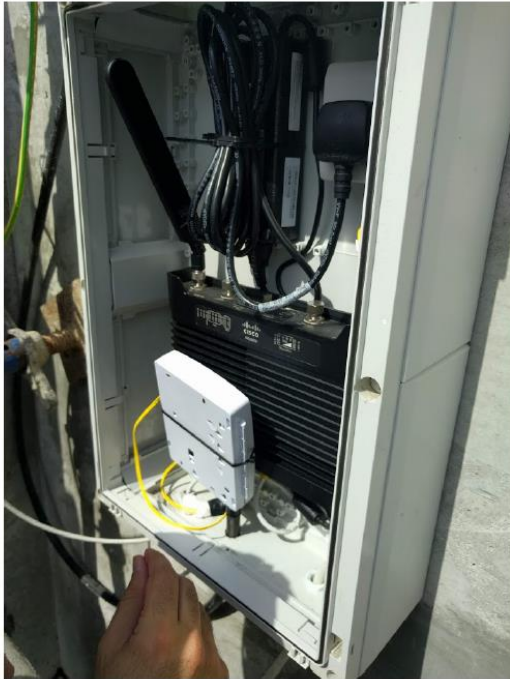
Cisco router in a cabinet
